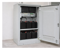
Demo battery backup
